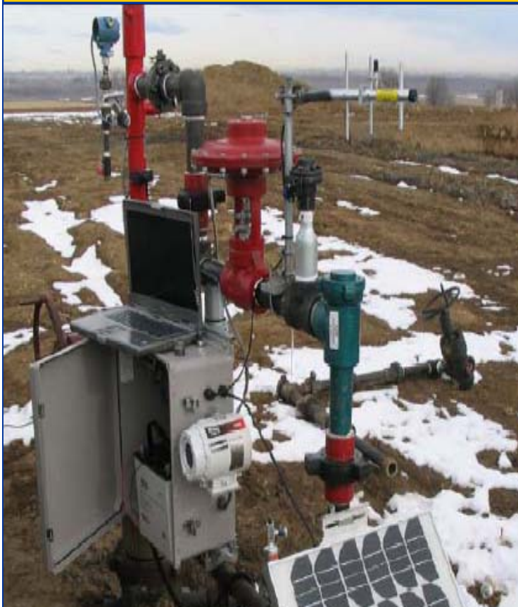
Exhibit 5: Typical Wellhead Equipment and Telemetry for Automated Control Systems for Plunger Lift
