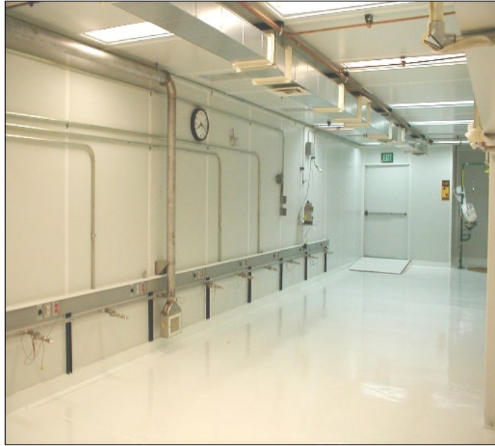
TA-3-29, Wing 9, Basement Room 9010, Process Code S01, Container Storage Process Code T04, Other Treatment
