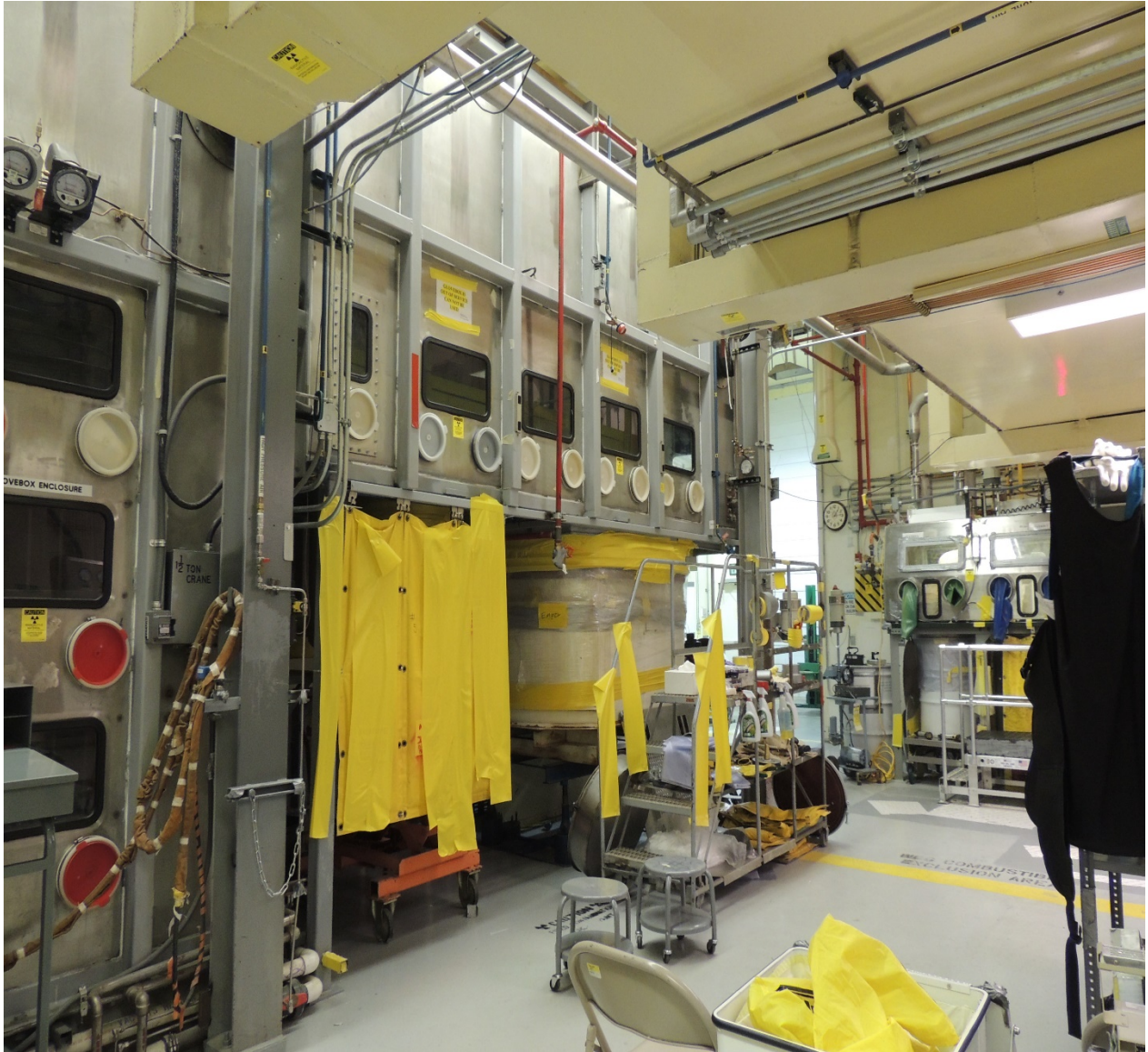
TA-50-69 Indoor, Rooms 102 and 103 Process Code S01, Container Storage Process Code T04, Other Treatment
