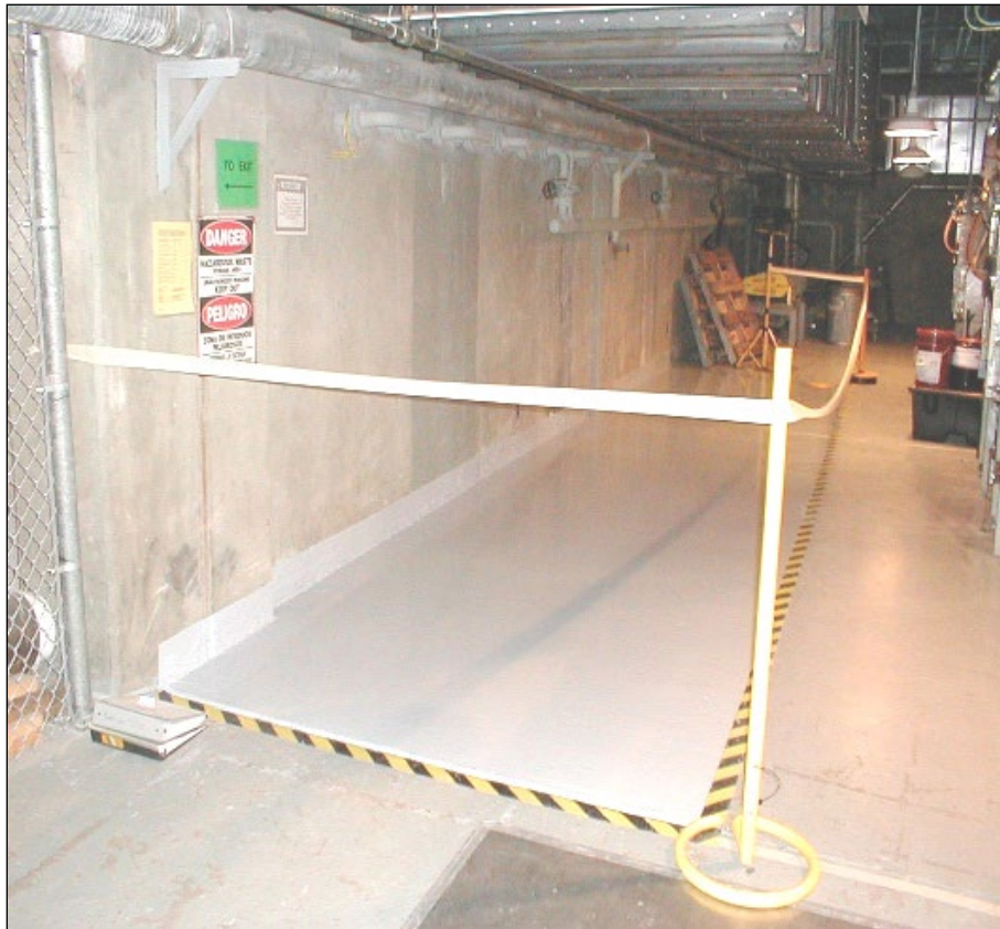
TA-3-29, Wing 9, Basement Room 9030, Process Code S01, Container Storage Process Code T04, Other Treatment
