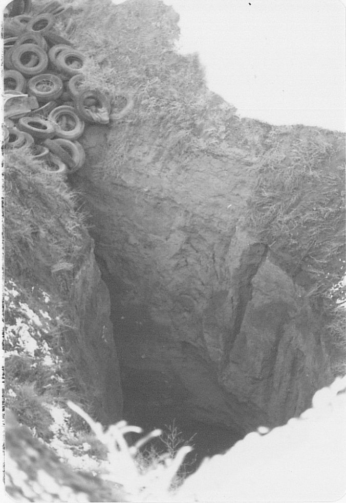
Photo (c) Close-up of lower portion of caved depression where it funnels into the old shaft.
