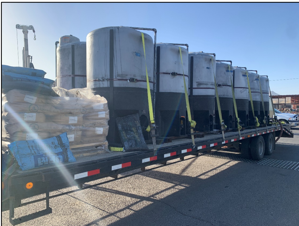
Photo 4. Injection solution tanks, bags of bentonite, and cold-patch asphalt.
