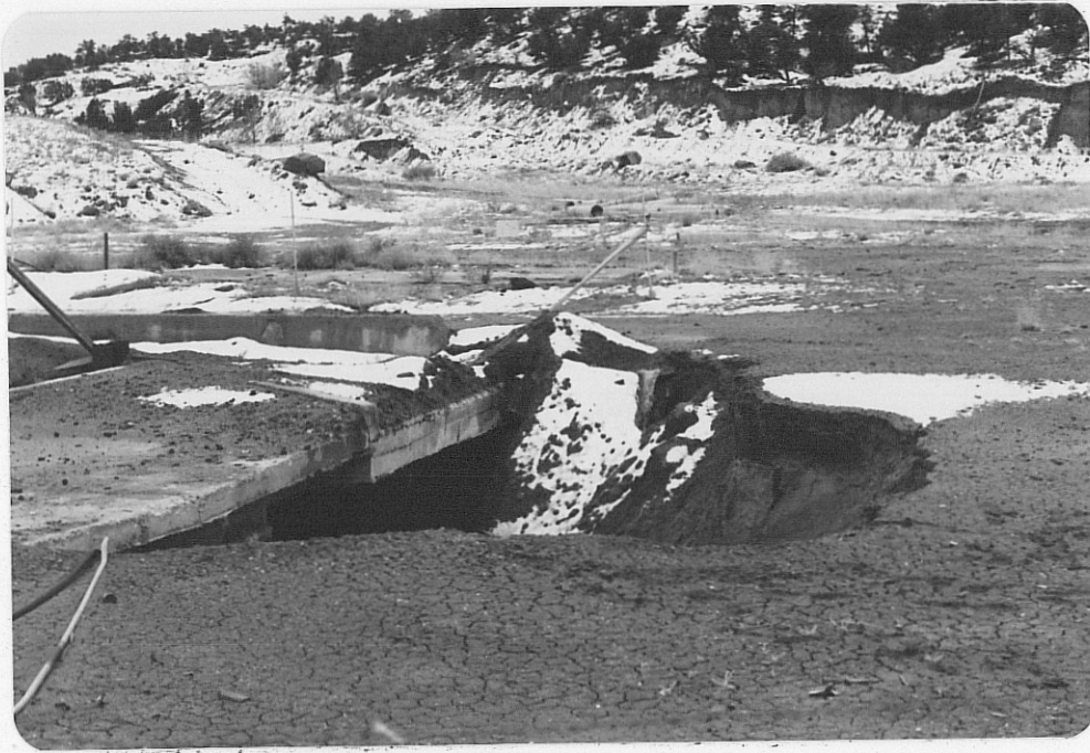
Photo (c) Close-up of shaft site showing extent of caving; concrete slab is 8" thick at far left.
