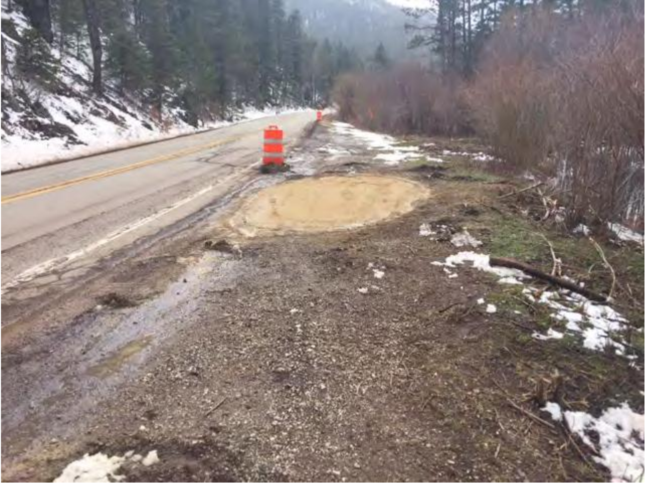
Photo 7 Backfill of area between edge of road shoulder and river south of Area #1.
