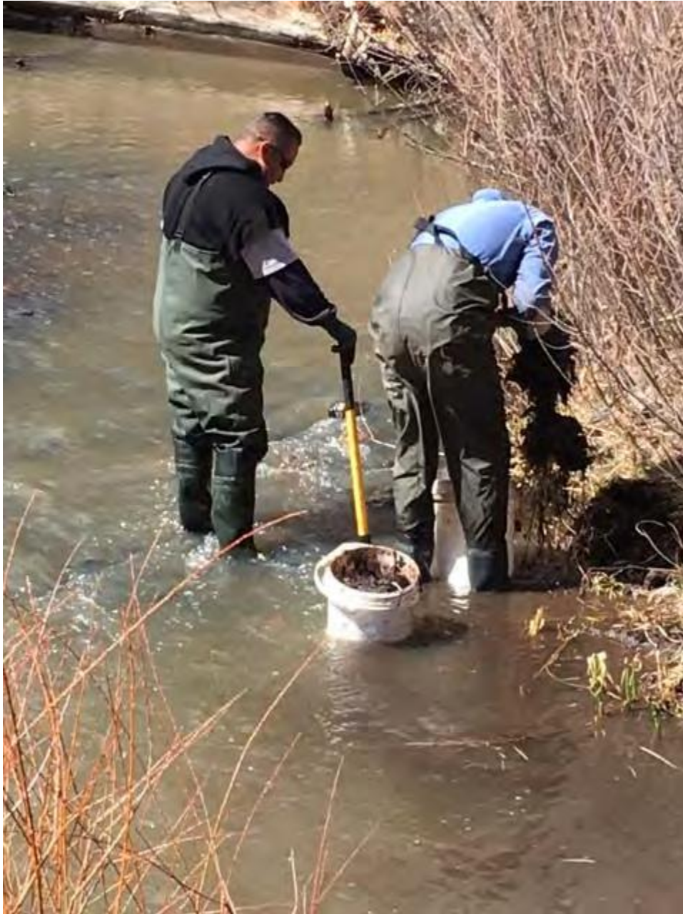
Photo 3 Use of buckets to transfer removed soils from the river bank at Area 2.
