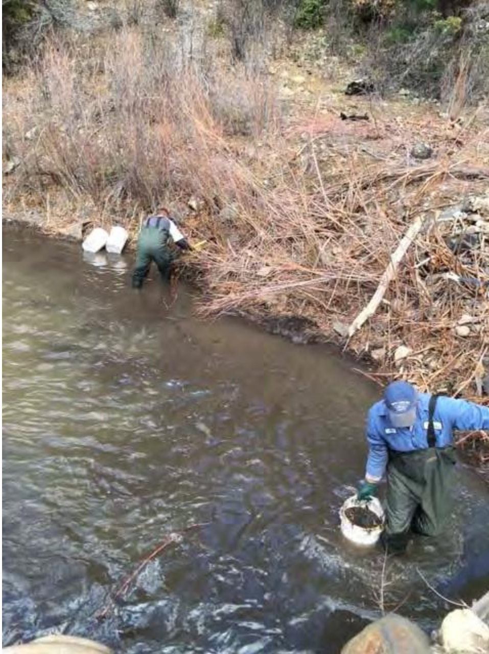
Photo 4 Use of hand tools and buckets to remove and transfer soils from the river bank at Area #3.
