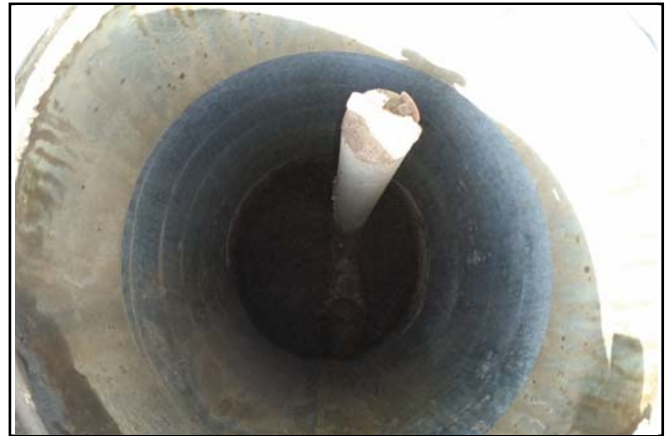
Picture 4 - Looking down into MW-4 well vault.
