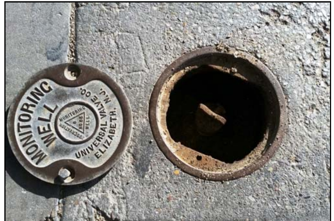
Picture 8 - Looking down into MW-8 well vault.
