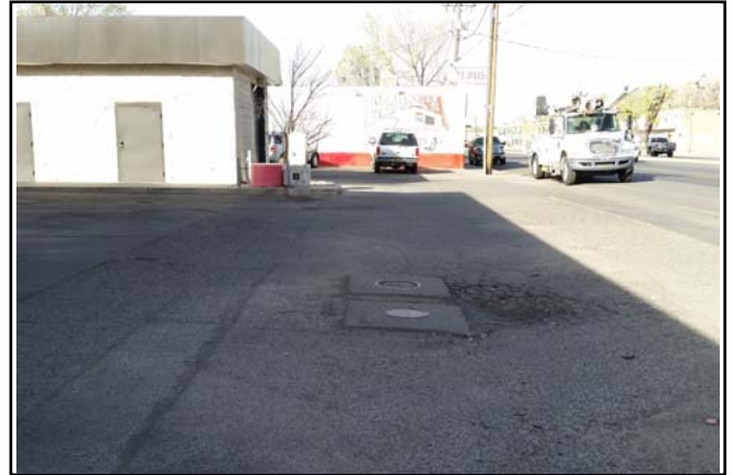
Picture 14 - Looking south at VP-5 well vault. The plugged and abandoned air sparge well (AS-5) is west of VP-5. Surface runoff water appears to infiltrate into the well vault from the depression.
