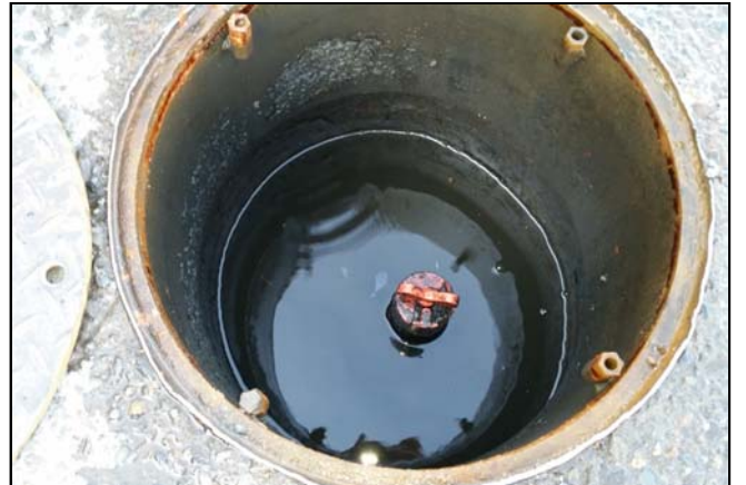
Picture 16 - Looking down into VP-5 well vault after bailing out water. WT believes that surface runoff water did not enter the well itself because the well cap appeared watertight.
