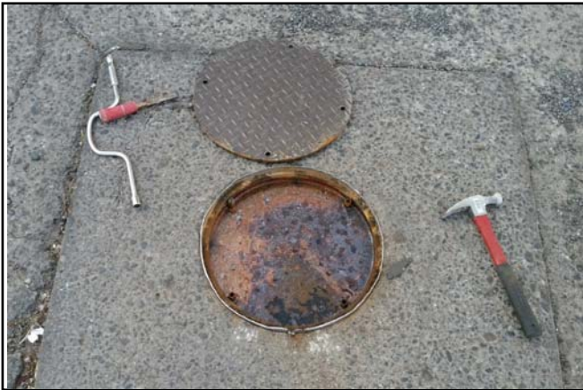
Picture 15 - Looking down into VP-5 well vault before bailing out water. The well vault cover was difficult to remove because the well vault rim was curled over the well vault cover.
