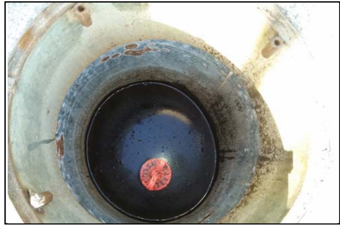
Picture 10 - Looking down into MW-9 well vault.
