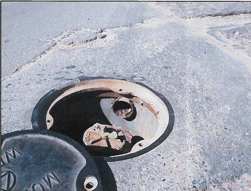
PHOTO 4 - MONITOR WELL W-3 CONVEYANCE PIPING BETWEEN WELLS.
