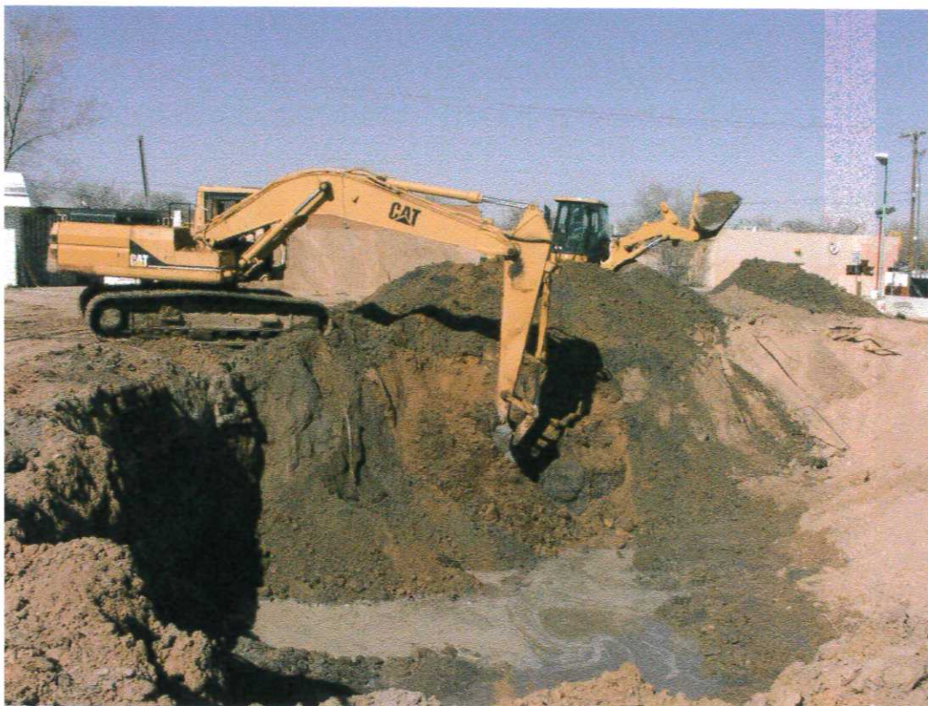
Photo 15. Removal and stockpiling of contaminated soil at southwest corner of excavation area.
