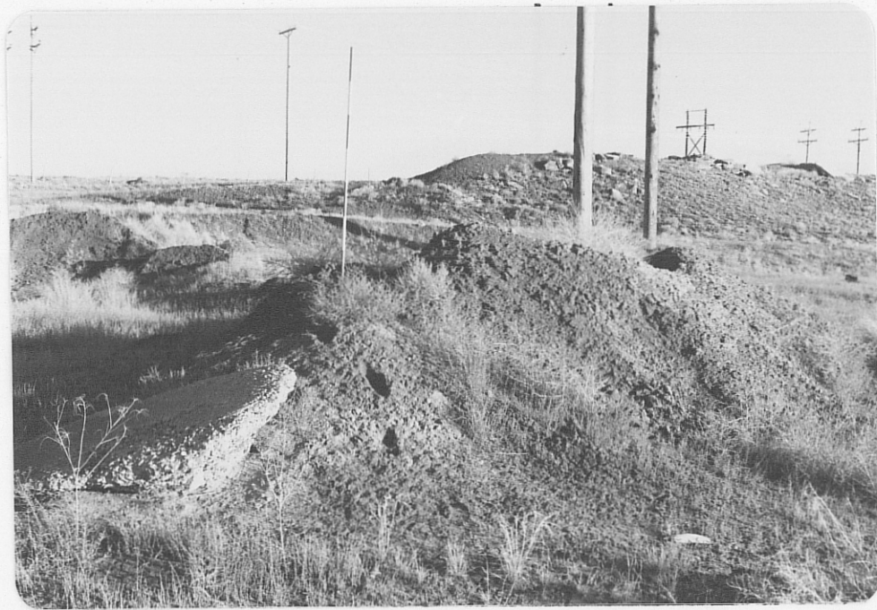
Photo (b) Looking southeast at mine shaft site which shows collapse features; note range pole for scale.
