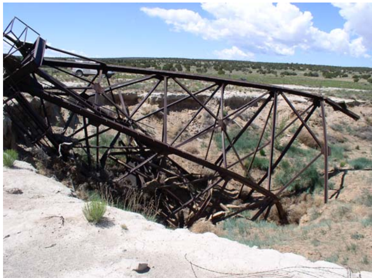
P1: Spencer Mine headframe collapsed into shaft due to arroyo capture and undercutting
