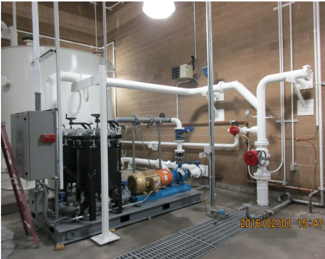
Influent tank and bag filters at GWTS
