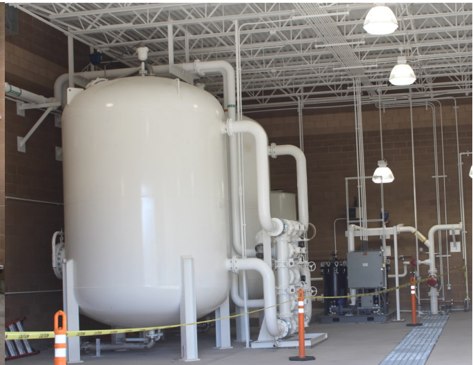
Two 20,000 pound carbon treatment vessels
