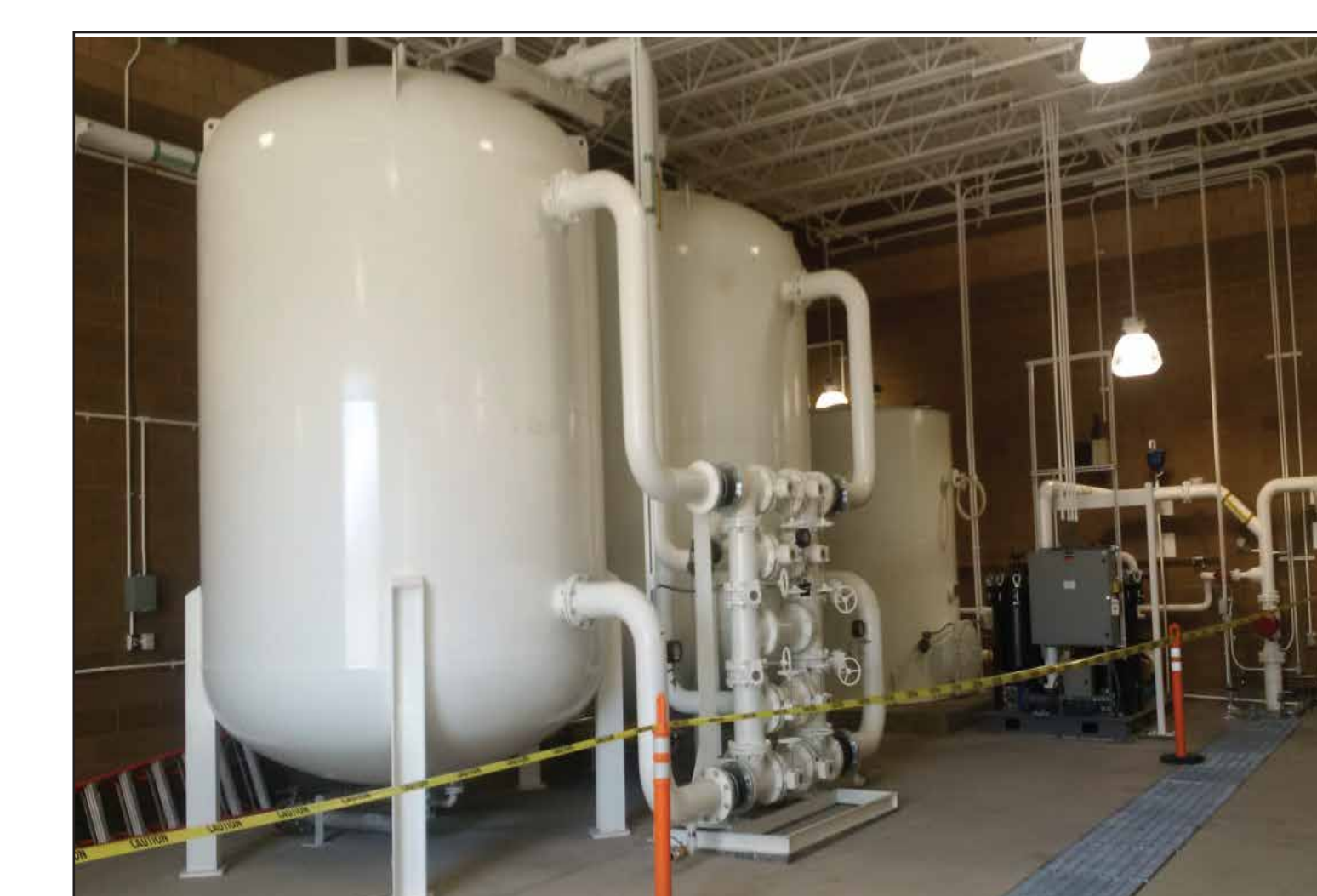
Granular activated carbon tanks used to treat contaminated water extracted from the plume.
