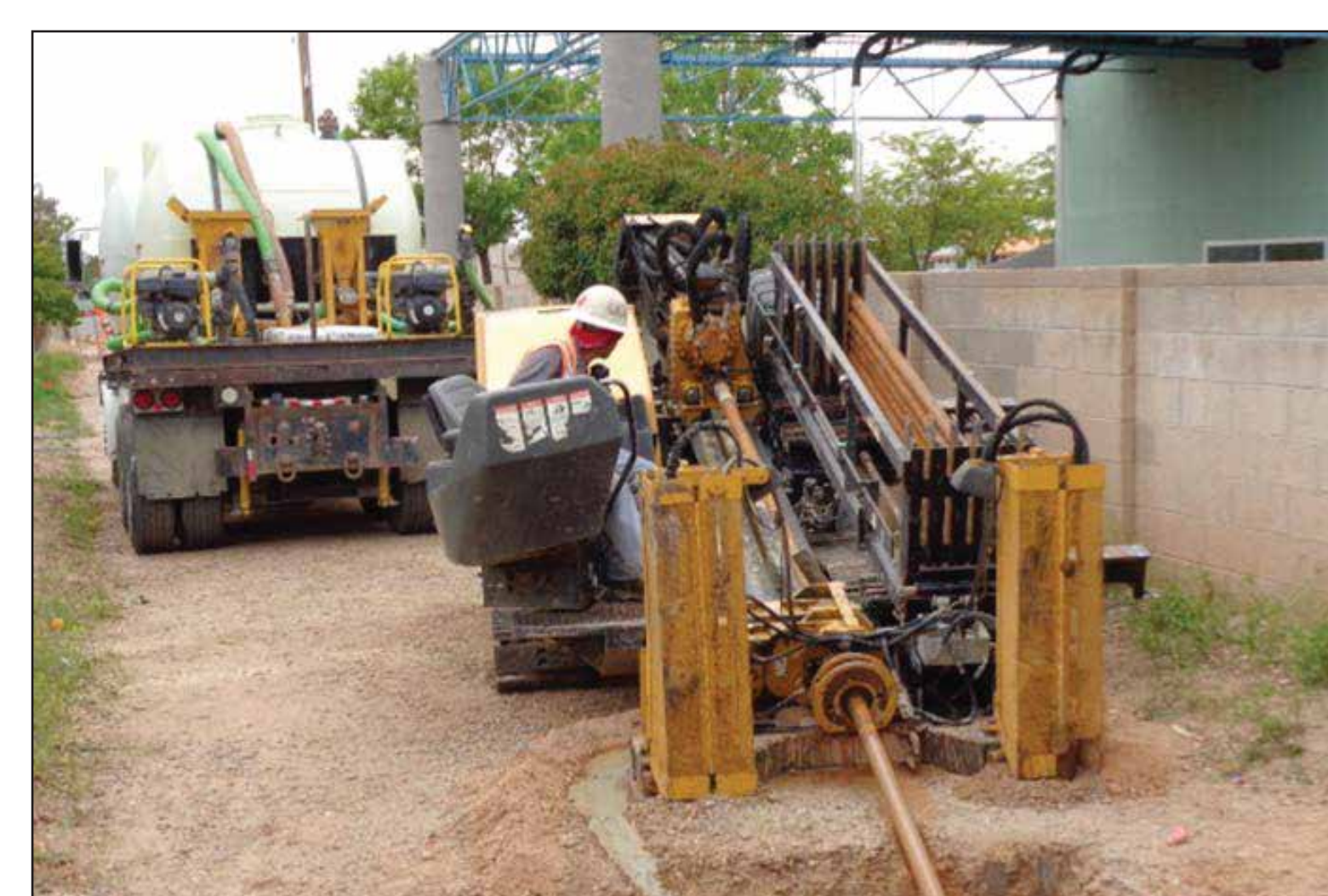
Directional drilling for installation of underground HDPE piping from extraction well KAFB-106228 to Kirtland AFB.
