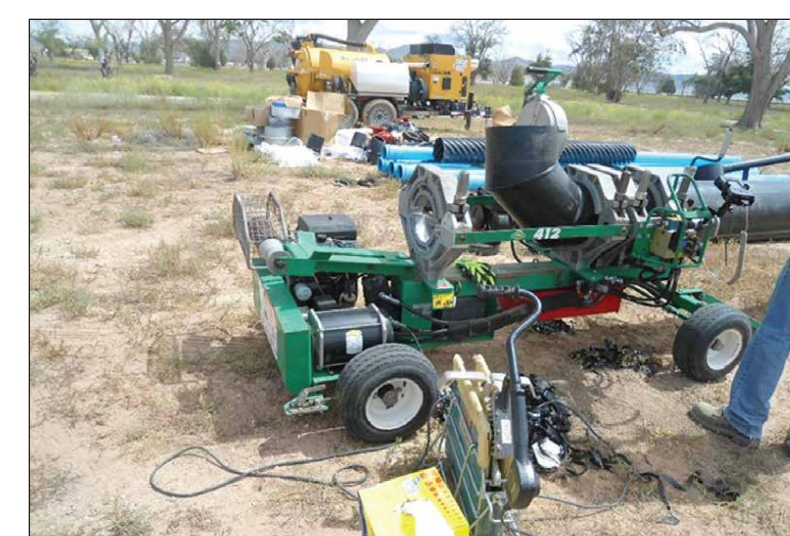
Fusing of the HDPE influent piping. This piping is being installed beneath the ground surface and connects the existing valve vault to the full-scale treatment building.
