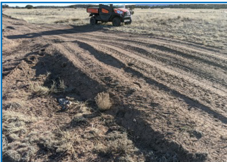
Example rolling dip. Rolling dips direct flow off of low-standard rural roads, reducing erosion of the road's surface and reducing delivery of sediment and nutrients to adjacent landscapes.
