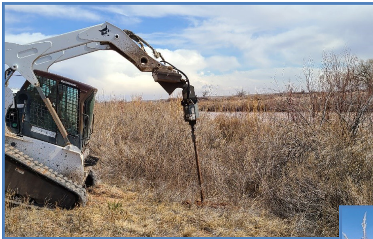
Photo left; Bobcat augers holes to plant cut Cottonwood tree poles down below the groundwater table on the banks of the Pecos River.
