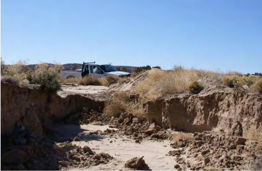
Example of gully erosion from a road, BLM lands, Alcalde, NM. 2007. J. Johnston.
