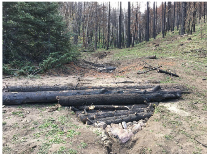
b) Post Fire Rehabilitation of the Rio en Medio: The completed structure.
