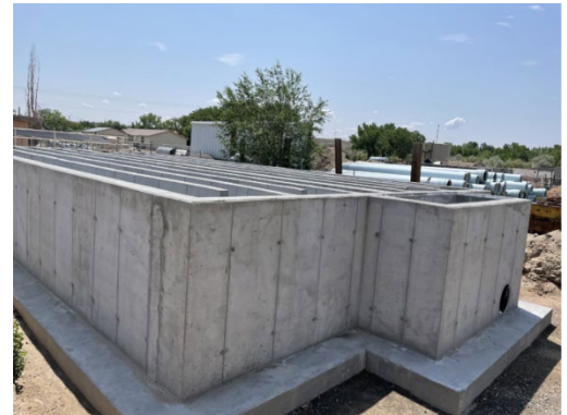
Chlorine Contact Chamber City of Bloomfield CWSRF 103
