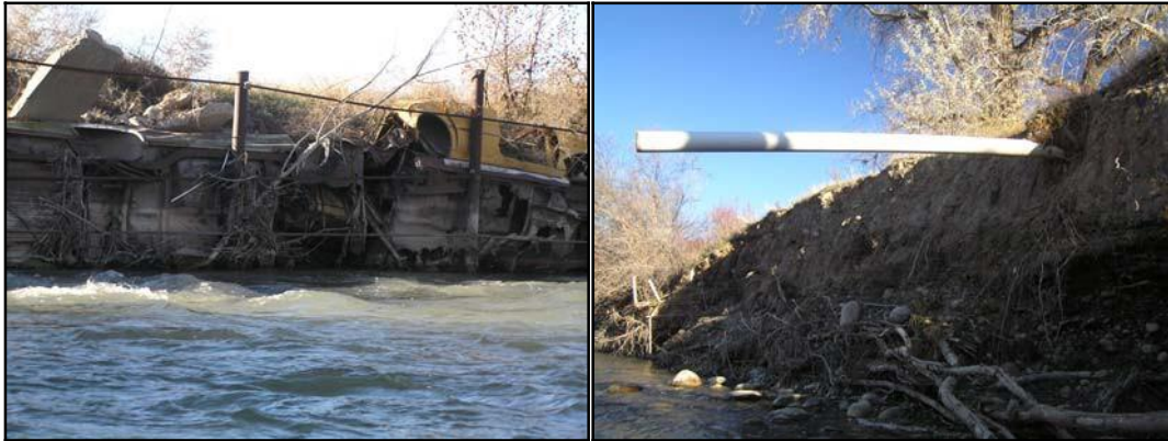
Figure 17. Picture of inappropriate bank stabilization (L) and actively eroding bank (R)
